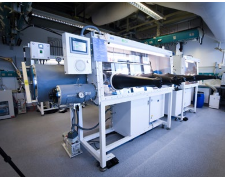
Glovebox facilities in the Bianchini group to assemble Li-ion and Na-ion batteries
